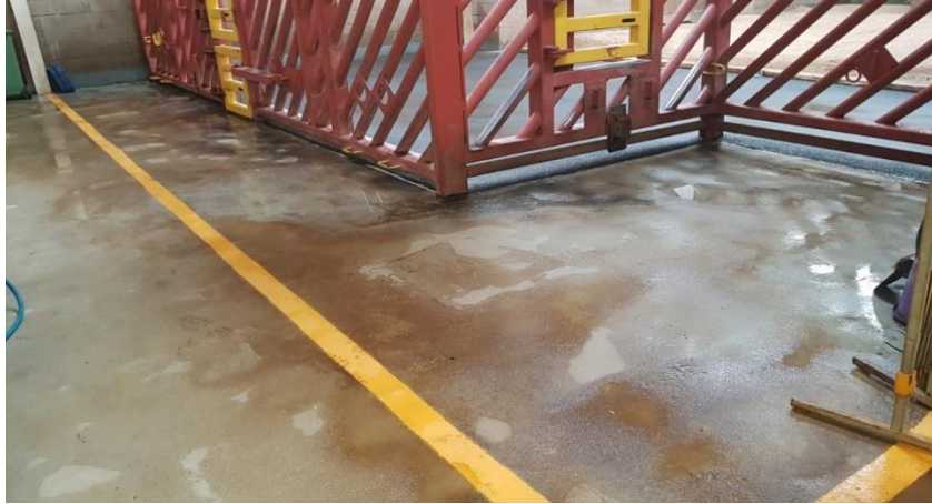
Figure 26 Clear lines of demarcation around the PC wall
